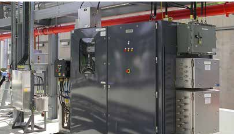
Exp Electrical Panel at BAE
